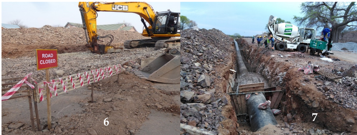
Photo (6) shows the excavations for the pipeline blocking the original entrance to the mission. The top of our church can just be seen above the rubble. Photo (7) shows the pipeline itself. This has forced us to make a new temporary entrance for the vehicles.
