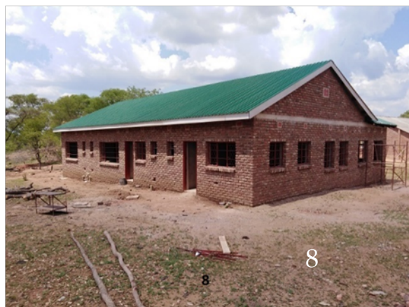
I hope the year 2023 will see an easing of the electricity shortages. Concerning our own projects, earlier this year we started building a new 4-bedroomed priest's house at St. Francis of Assisi Mission, Cross Dete. Photo (8) shows the roof is now on. This is a new mission, almost 100 Km from our mission.
